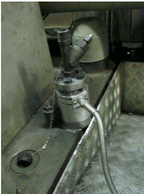
HTT-04® sensor mounted on a special designed adaptor for permanent installation on Wärtsilä 46 engine
